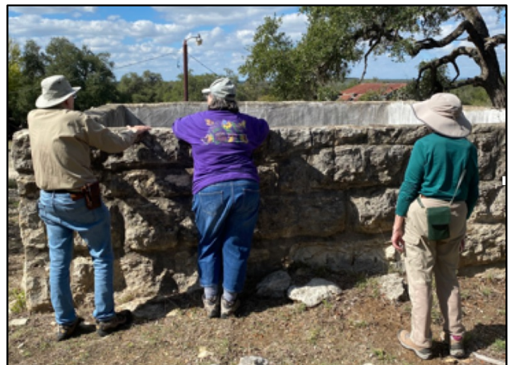
The cistern, now missing its metal roof.
