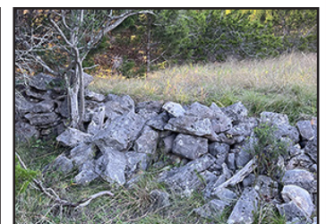
Fig. 5. Soil build-up behind wall. Photo by Mackenzie Brown
