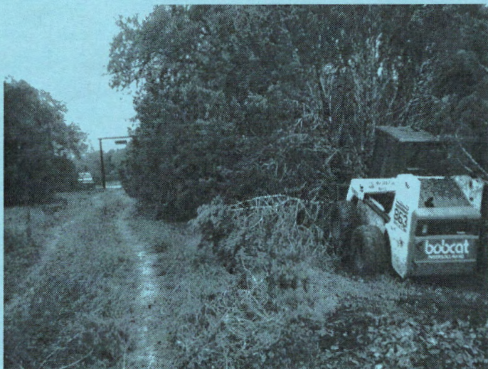
A.J. Brunner operating the Urban Concrete bobcat clearing the entrance to the Northshore of Guadalupe River State Park.
